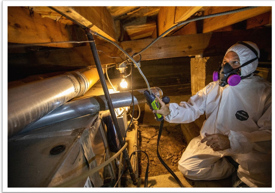
Ron Piz, quality control inspector auditor, and furnace technician, for the Energy Resource Center tests for gas leaks and performs combustion analysis in the crawl space of a home in Denver, Colorado. (Photo by Werner Slocum / NREL)
