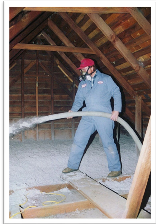
A technician insulates the attic space of a home to improve its energy efficiency. (Photo by Community Services Consortium/NREL)
